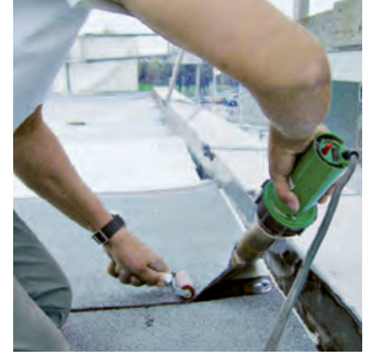
Welding of bitumen sheeting using the powerful ELECTRON with a wide slot nozzle.
