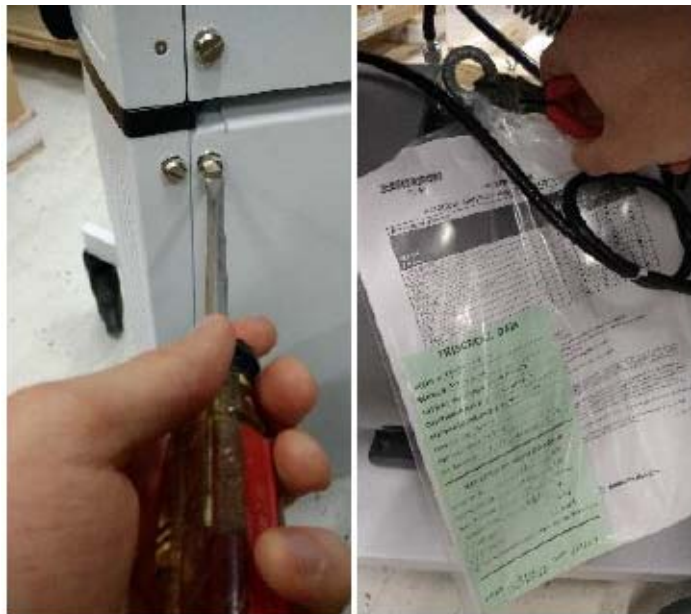
Figure 1-7 IDP-15 Rear Pump Access
