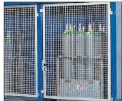
Lockable doors, either as mesh or fire-rated versions ensure that unauthorised persons have no access
