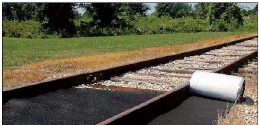
Use on railway lines: the wide roll fits snugly between the rails. Side areas are protected with the narrow roll.
