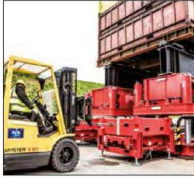
▼ A load is lifted in increments as barrels are slid into the system, lifted, and stacked; forming 'lifting towers'.
