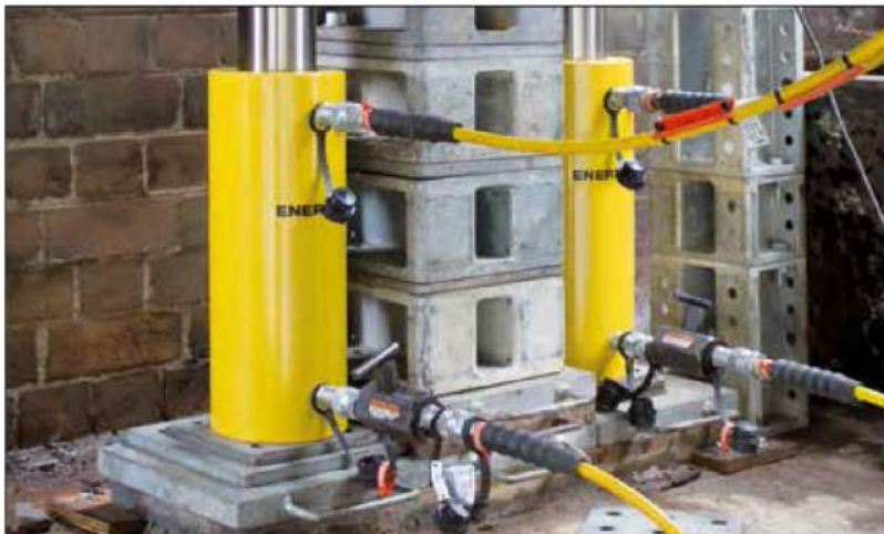
▼ Bridge maintenance: A 200 ton bridge was lifted using 8 cylinders to replace the old bearings.
