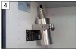
4 Fire suppression system
