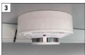
3 Smoke detector and temperature sensor
