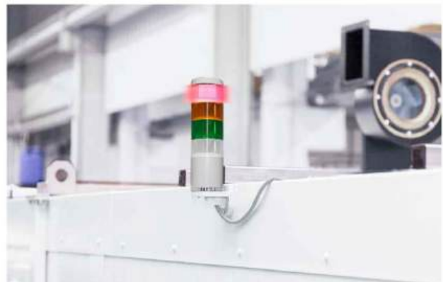
Alarm signaling by signal lamp (visible) and horn (audible).
