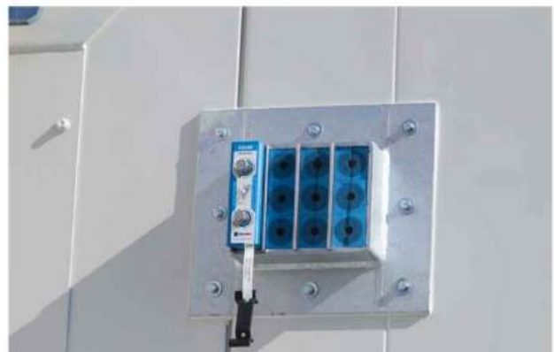
Passage of cables through the wall of the fire-rated store (fire bulkhead), while maintaining the fire resistance of the component.
