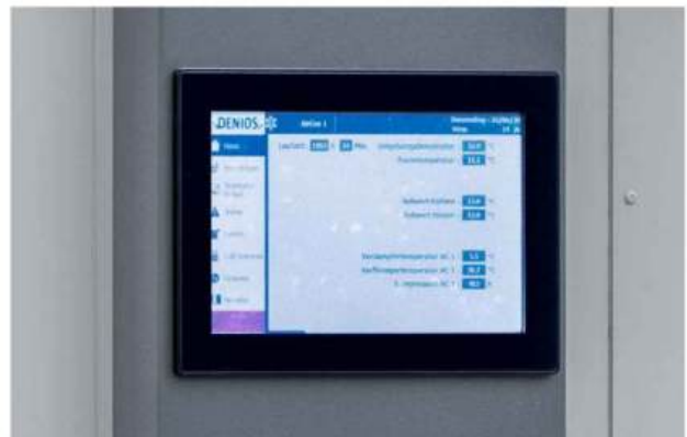
Central monitoring and control of all electrical components with the DENIOS Communication Bar.
