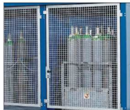
Lockable doors, either as mesh or fire-rated versions ensure that unauthorised persons have no access
