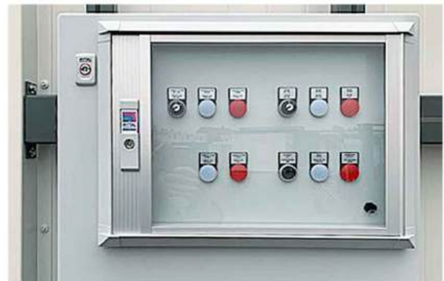
Enclosed user controls: controls and user controls are protected from unauthorised access in the front of the switch cabinet.
