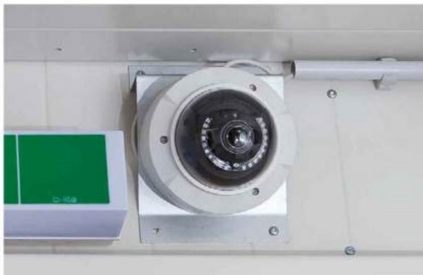
Video surveillance and recording of the hazard area indoors or outdoors.
