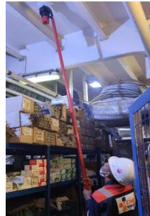
SMOKE DETECTION SYSTEM
